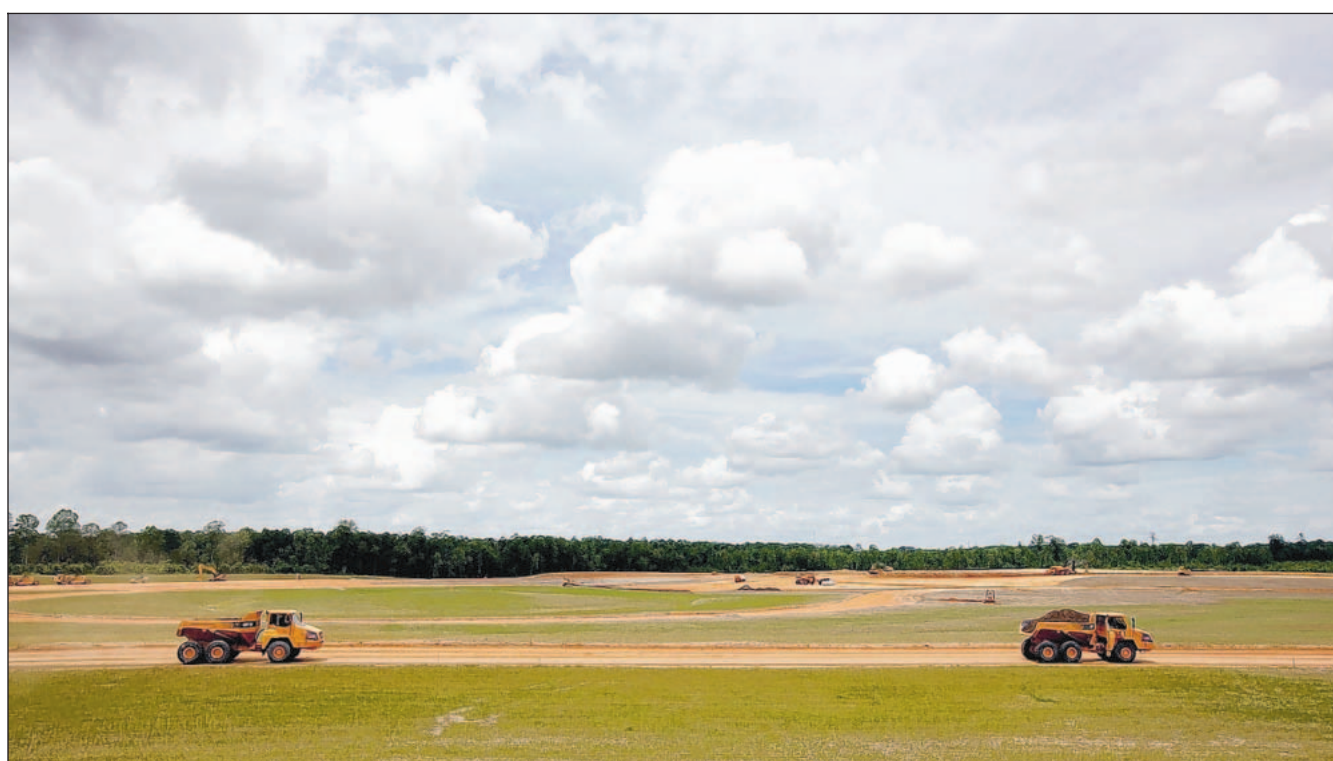
The N.C. Center for Automotive Research, under construction near Roanoke Rapids, got half of its $15 million in state money under the condition that a private partner promise to create jobs. That hasn't happened.
